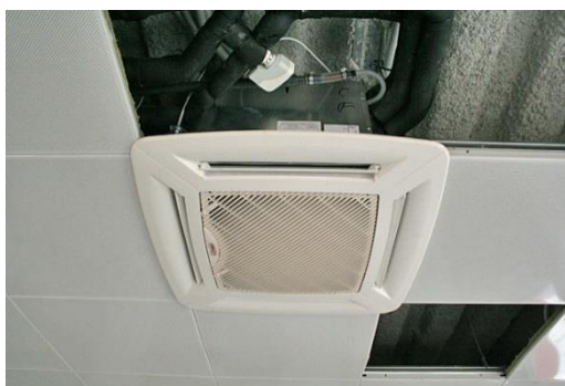
Figure 5-9: Split type fan coil (mounted on the false ceiling of the room)
