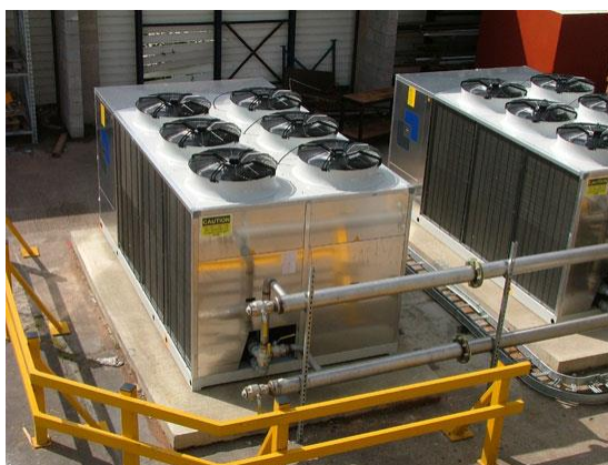
Figure 5-5: Cool water cooling plant. Air condensed water chillers.
