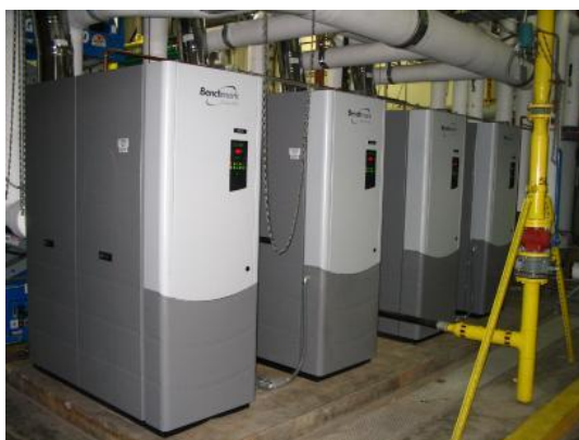
Figure 5-1: Hot water generation plant (condensing boilers)
